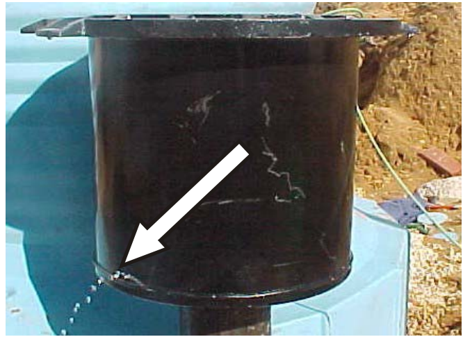
New spill bucket undergoing testing at a tank installation site. Arrow indicates water leaking out.
